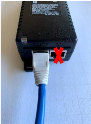
Figure 6: Ethernet cable connected to the power brick
